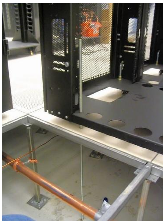
Figure 3 – Seismic safety for racks [source: Data centers lectures, Instituto Superior Technico Lisboa]
