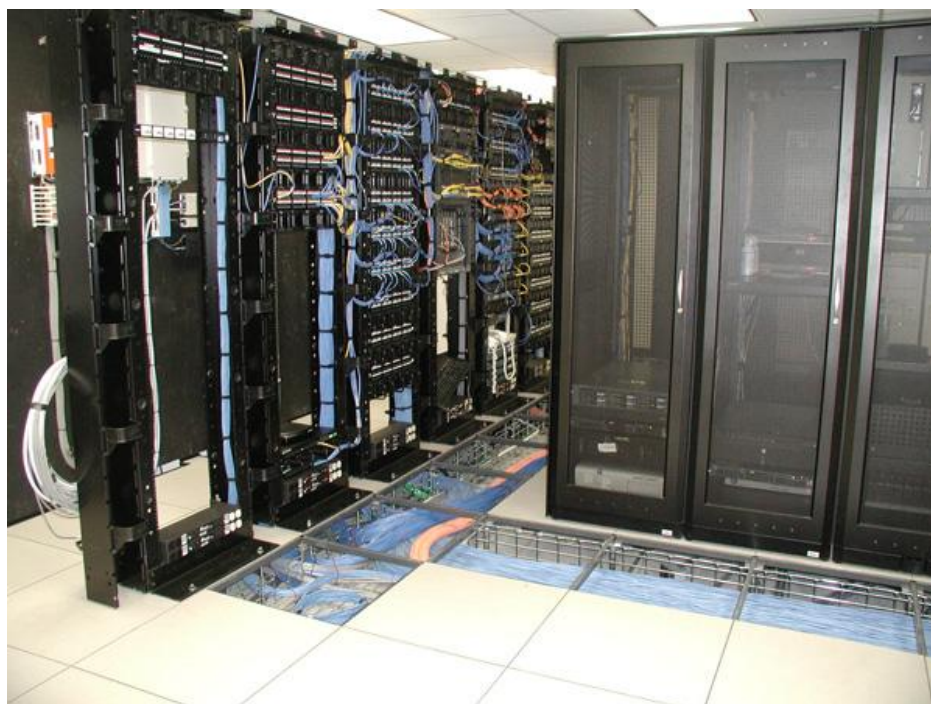
Figure 2- Raised floor in server room
