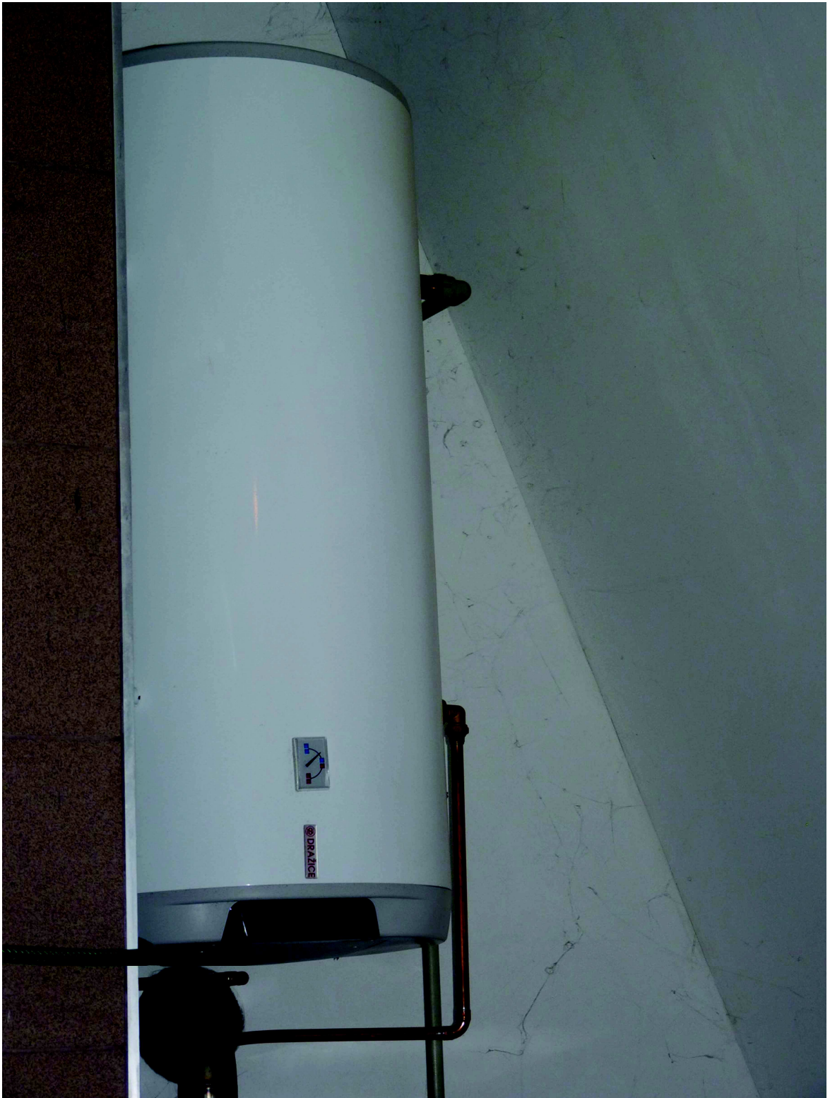
Boiler heated with cooling water, Appendix 8
