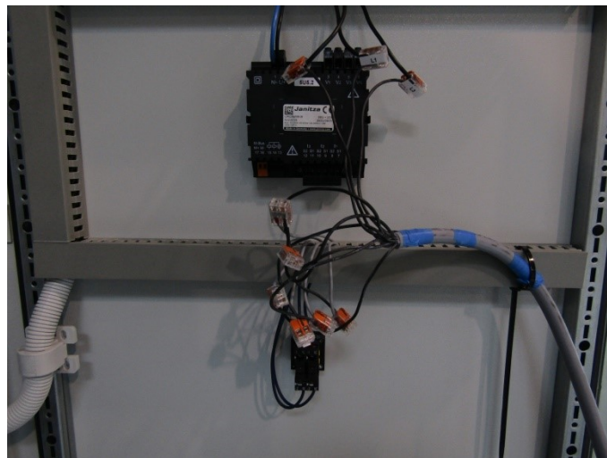
Figure 57: Electric connection of the energy meter to the welding cell distribution.
